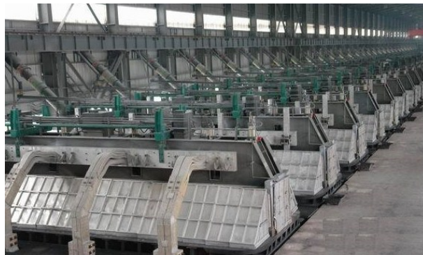
Figure 1 Electrolytic cells in an electrolytic aluminum plant.
